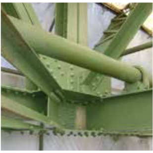
Bridge capital improvements such as painting were a major component of governmental fund activities
