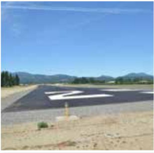
FAA mandated runway shift was completed in 2013 at the Ken Jernstedt Airfield
